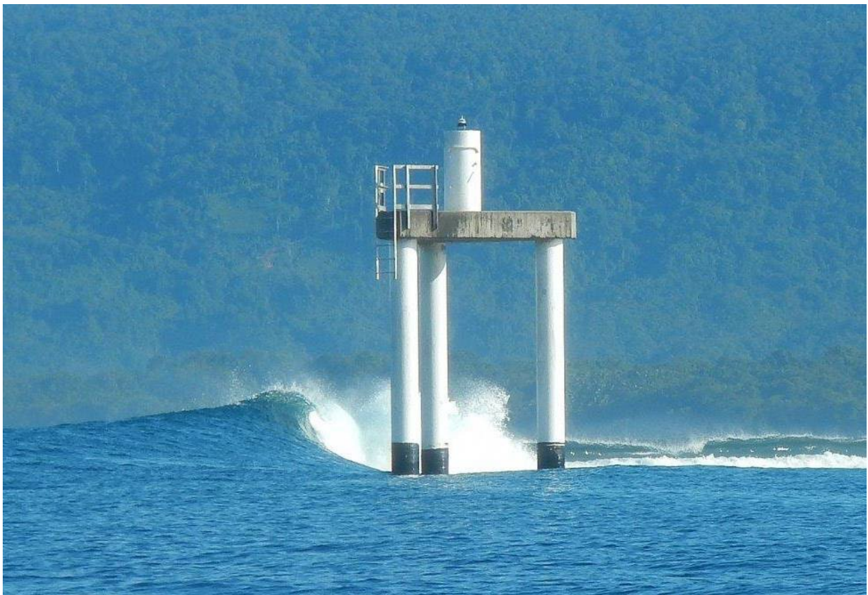
Figure 2 Example of multi-steel piled, concrete light platform with GRP light tower, access ladder and tape wrapped piles within the splash zone
